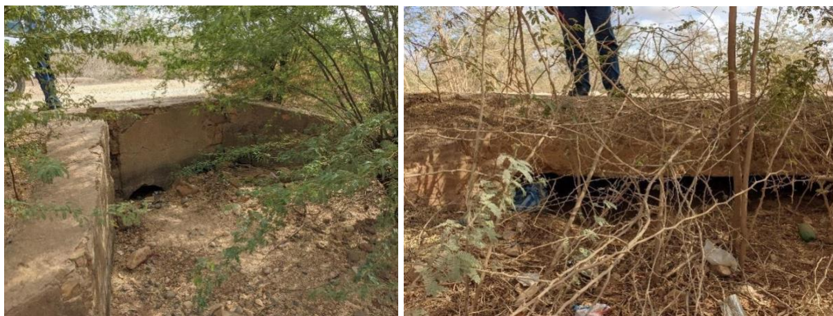
Figure 14 Sample photos of blocked drainage structures
