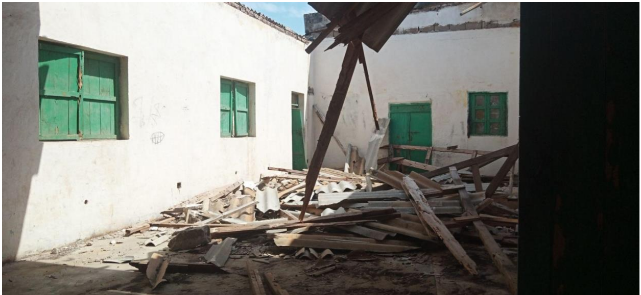
Figure 4-3: Collapsed roof in the admissions area.
