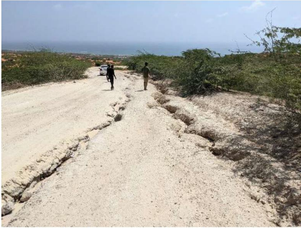
Figure 12 showing a section of the road with pronounced down cutting on the road surface. Note the lack of a side drain
